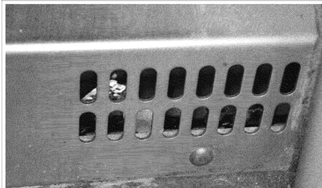
CLOSE UP OF AIR GRILL
